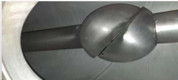
Stress Cone Fault (2012)
